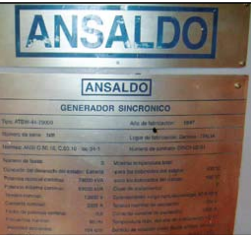
Picture: the Ansaldo generator installed in the Marcel Laniado de Wind hydropower plant. Source: CAIC's technical group.
